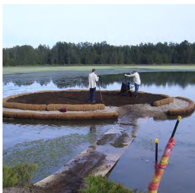
Constructed earthen and floating islands provide safe roosts and breeding sites for waterbirds
