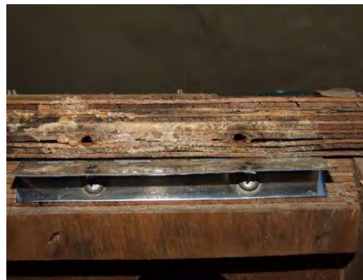
Figure 3. Decay around hinge screws will result in the lid falling off
